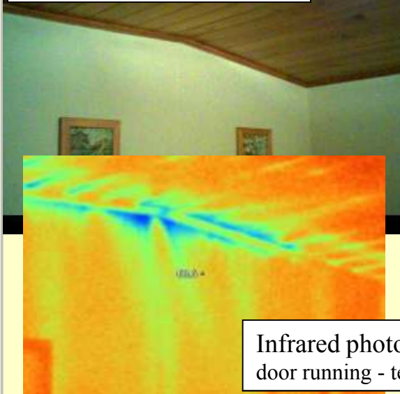
Incorrect - shows high leakage under negative pressure test
